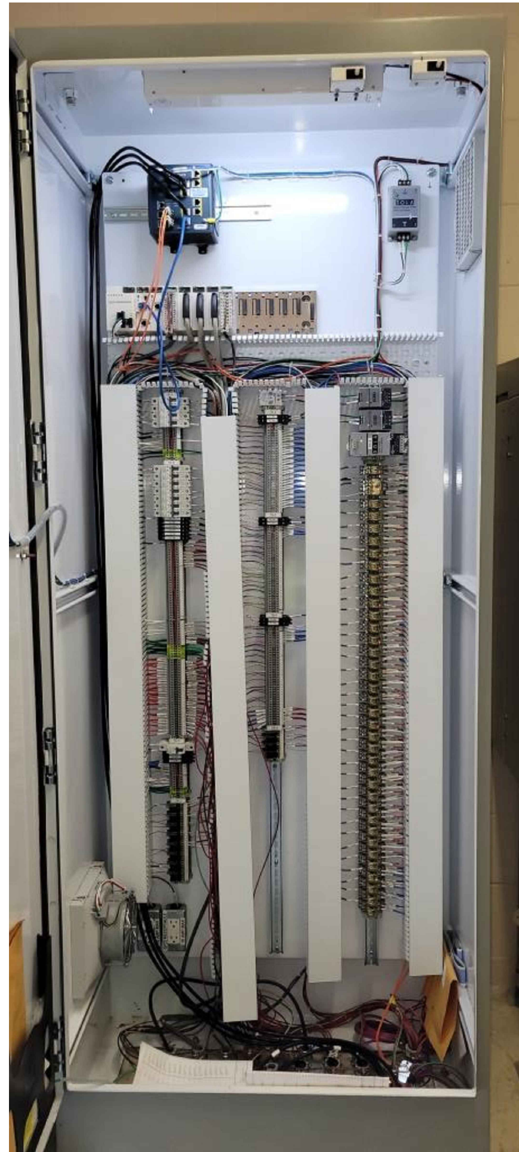
EXISTING MAR-SHB-PLC ENCLOSURE INTERIOR PHOTOGRAPH 1
